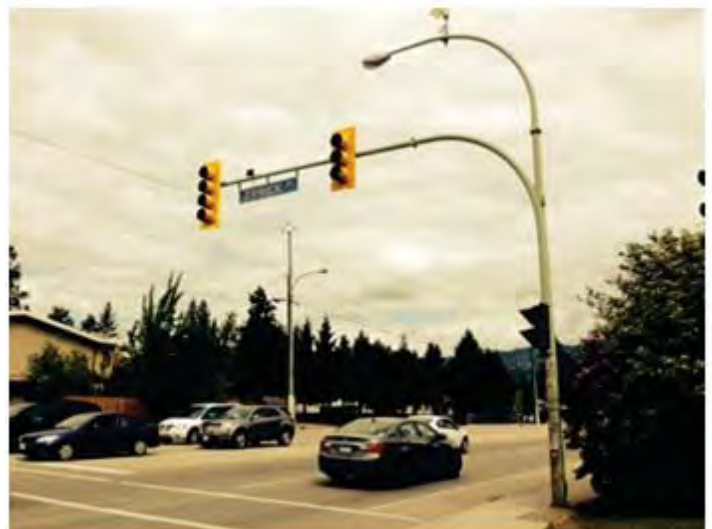
Radar unit on the pole
